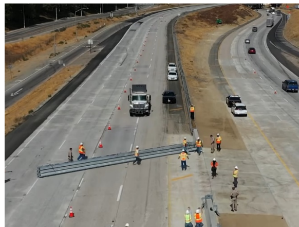
Figure 89. A median turnaround gate installed on the I-5 Grapevine at the Tejon Pass in Los Angeles. The gate allows Caltrans to create a turnaround for vehicles, including large trucks, when snow closes the pass. Alongside “Operation Snowflake” the gate is part of a coordinated strategy to reduce closures and avoid congestion when closures occur. Source: Caltrans 2020.
