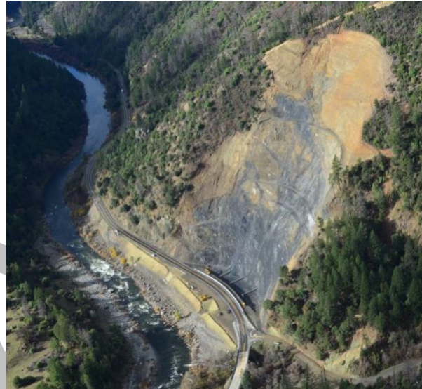
Figure 9. Landslide on Highway 299 near Big French Creek in Trinity County. Highway 299 was closed for several weeks to repair the road and construct a new catchment for future landslides (area between the slope and the road). Source: Caltrans 2018b.
